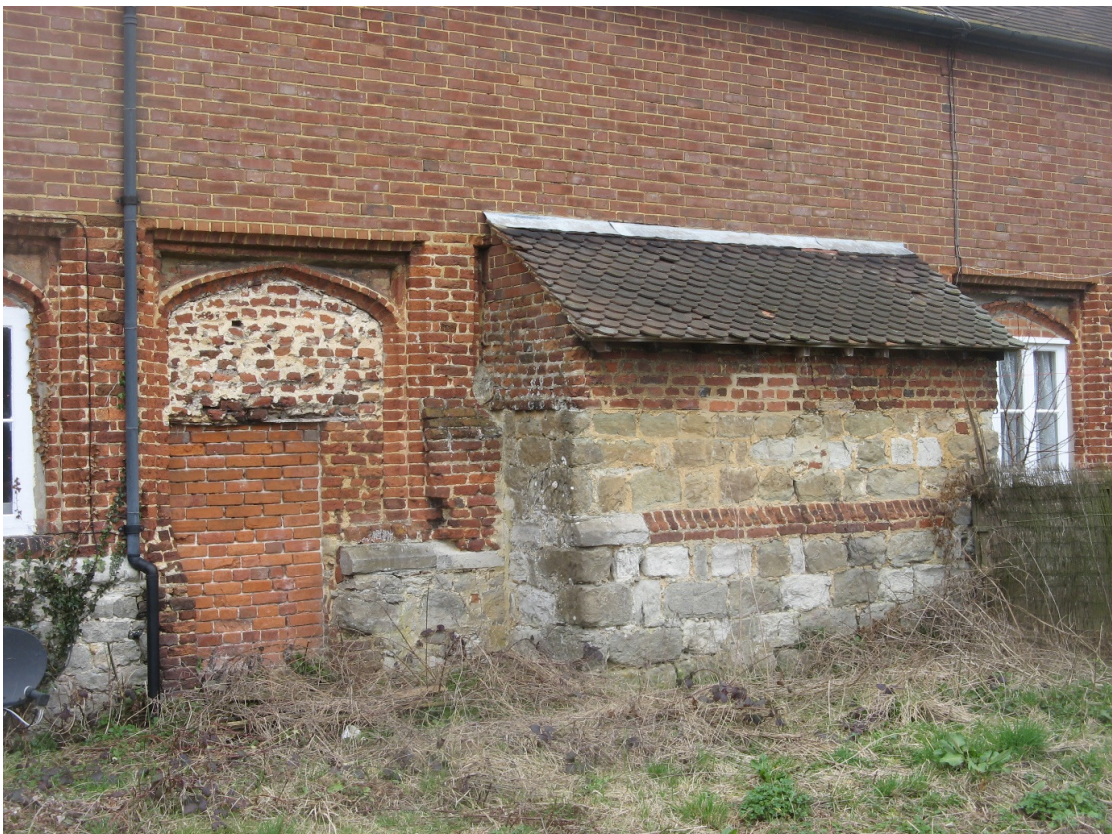
Fig 17 The projection on the south side of the north-west range; note the section of the plinth raised in brick, and the chamfered jamb of a doorway formed through one of the arched openings of the cloister. The rough infill above it is of uncertain date, the infill of the doorway around 1800
