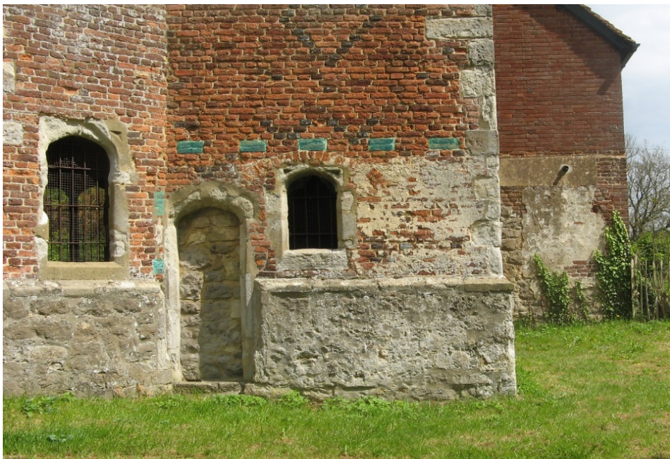
Fig 18 The south side of the garderobe tower showing blocked sockets for rafters, and probably rails of timber-framed wall, and internal plaster on the formerly external wall
