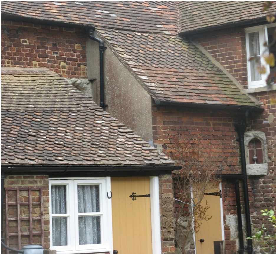
Fig 16 The remains of the added garderobe tower – the doorway is a 20 th century insertion
